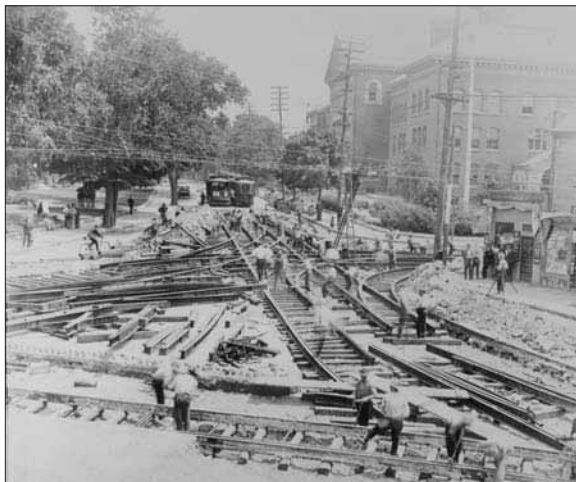
Trolley track construction Malden, MA , 1902. (Photo courtesy of the Boston Public Library, Print Department)
